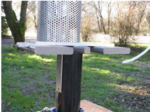
Pump on 4" surround with brace fully retracted and pump supported on 1" shim.
